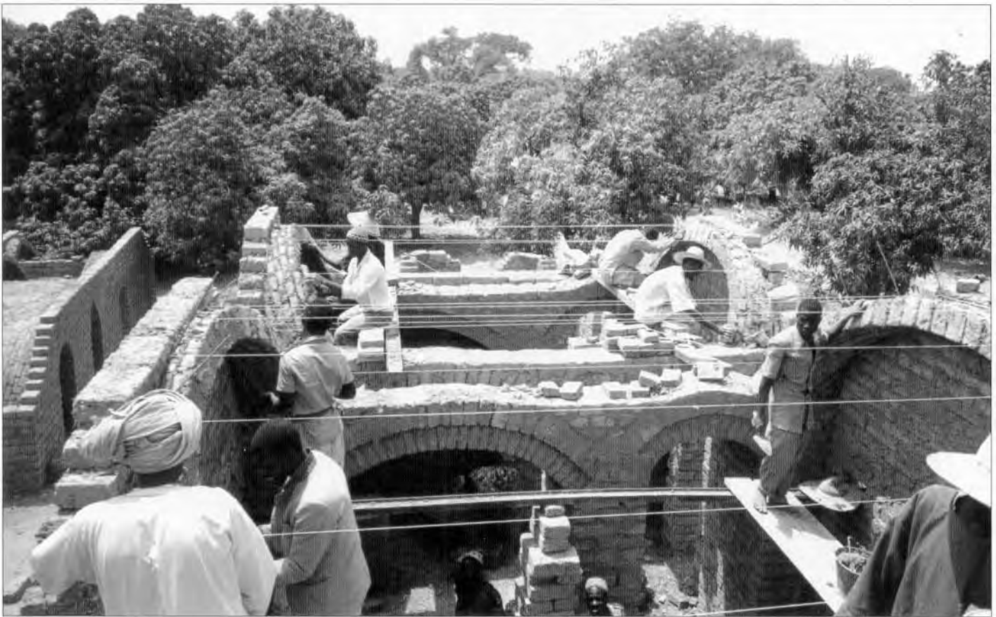
Figure 2 “Alcove” building under construction. Note the use of strings as a guide, the practice of starting the vault from both ends simultaneously, the use of off-centred vaults and open arches to create a spacious interior.
