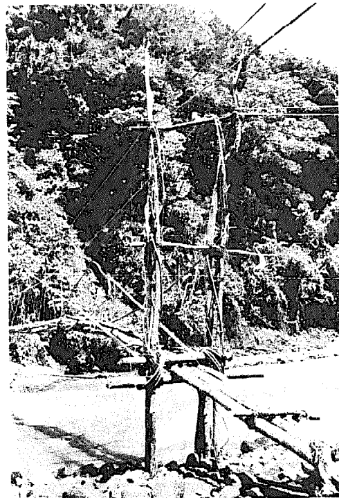
Fig. 136 West pylon, Gumbum Bridge. Note the holdback cables at the top and the abutment and cantilever design at the bottom.
