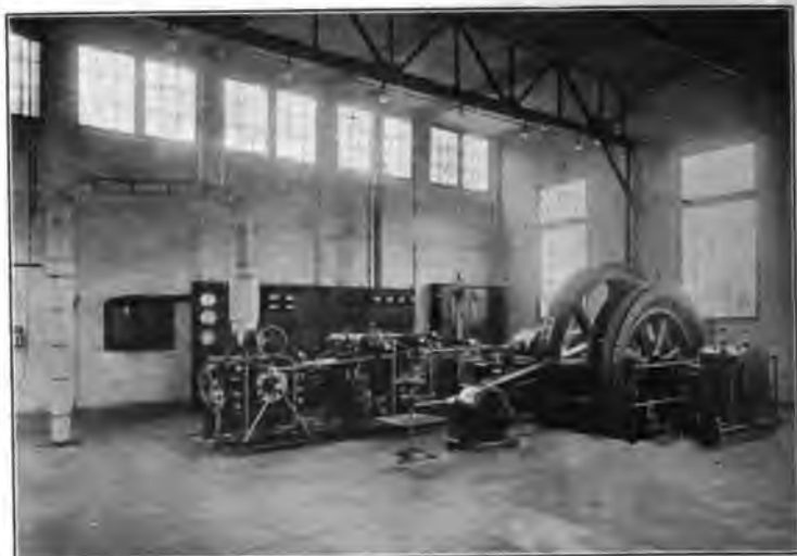
FIG. 289.—Compound Corliss engine connected directly to an a-c. generator. Belt-driven exciter in front, switchboard in rear.
