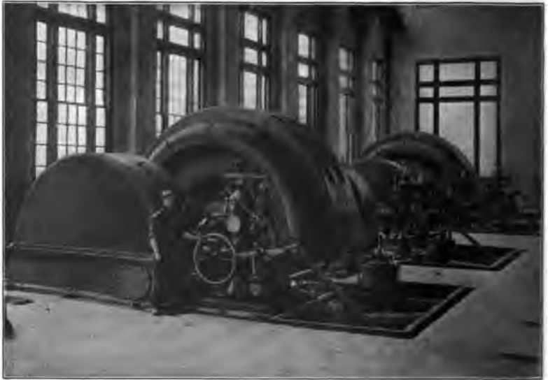
FIG. 292. — Big Creek Development. Power station No. 1. Hydraulic head 1900 feet. Two 17,500-kv-a. 6600-volt generators, each having a momentary peak capacity of 25,000 kv-a. Apparatus controlling Pelton water wheel in foreground.
