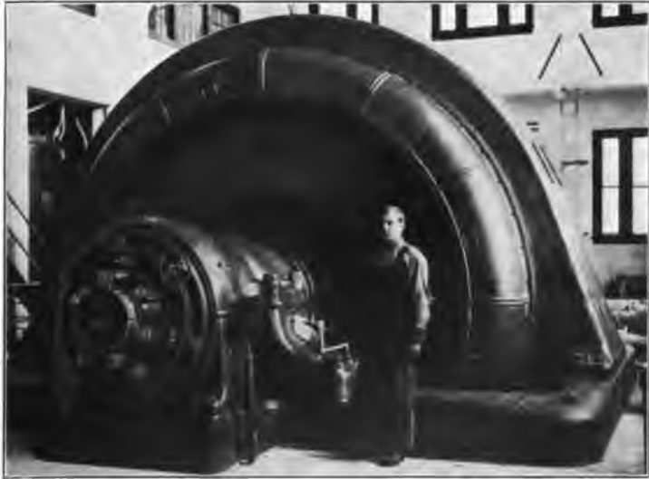
FIG. 280. — Synchronous condenser in substation at Eagle Rock, California, used to improve power factor on a very long transmission line. The exciter is in the foreground.
