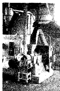
Briquetter, Screw-Conveyor & Dried material Pool
