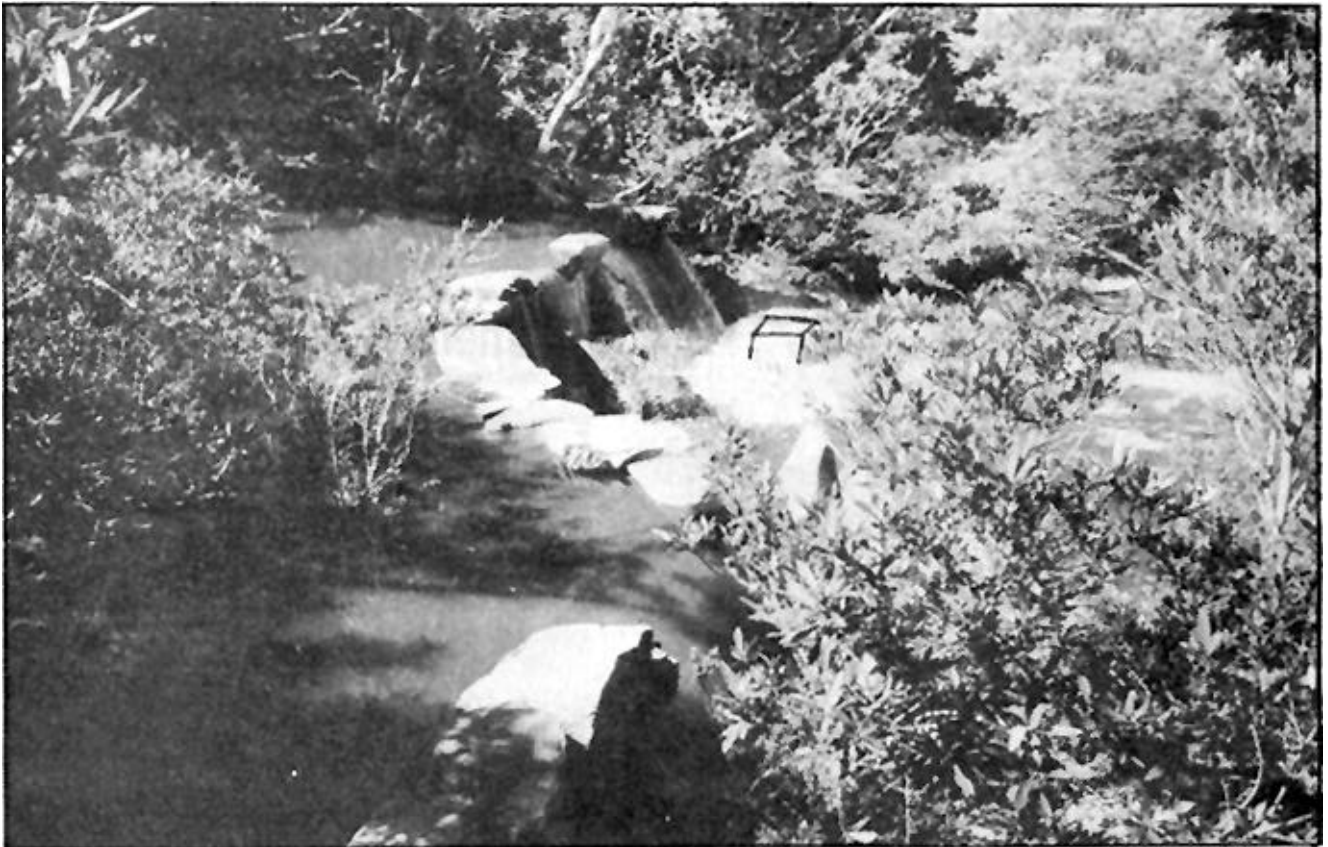
The pump and turbine were unaffected by this flood which totally submerged them both. The top half of the pump box is visible in the centre of the photo.
