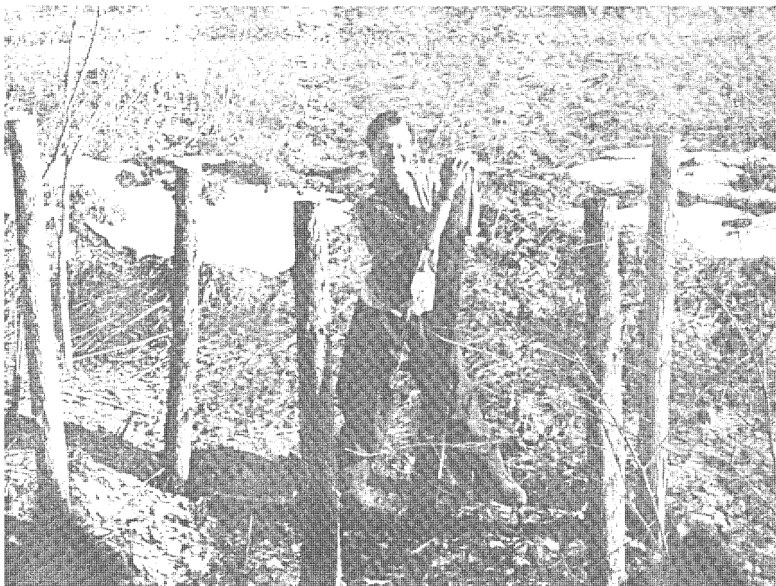
A YOUNG LADY SETTING CEDAR POSTS IN THE GROUND FOR THE CONSTRUCTION OF A DOUBLE-CHAMBERED COMPOST BIN.
