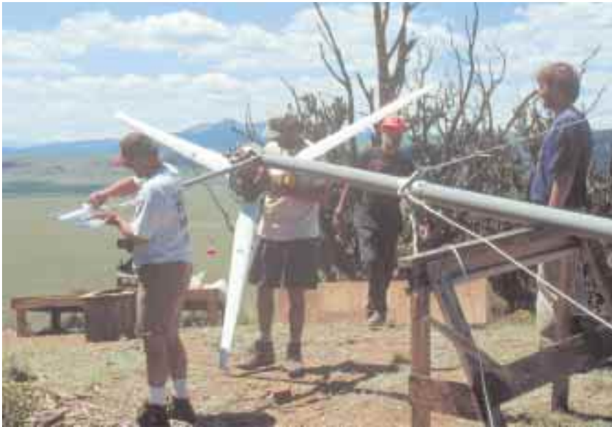
Final nuts and bolts check on the Whisper H1500 before we raise the tower.
