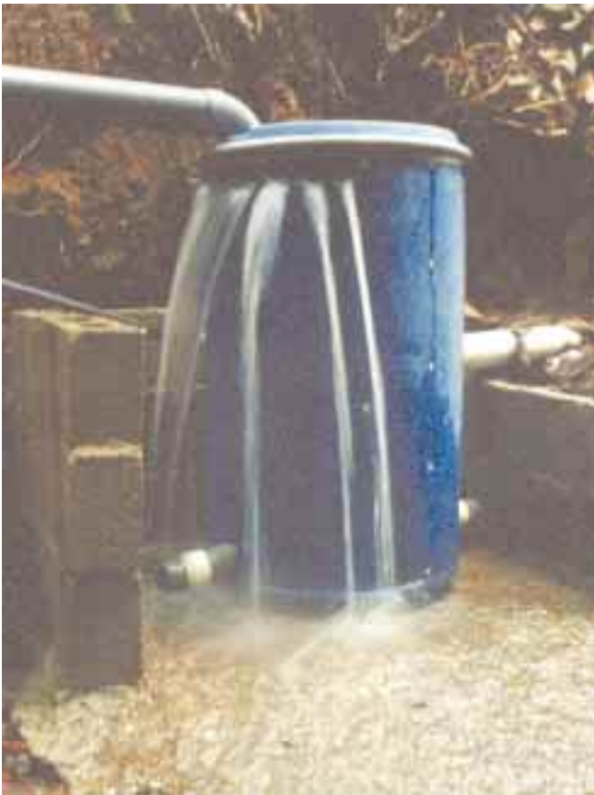
German Llano's filter tank, at the top of 55 feet of head, provides a clean 73 gallons per minute.
