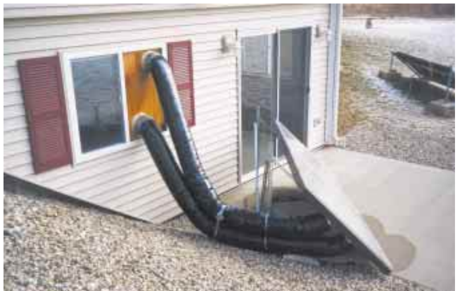
Back of the solar collector showing part of the support structure, as well as insulated cold and hot air ducts.
