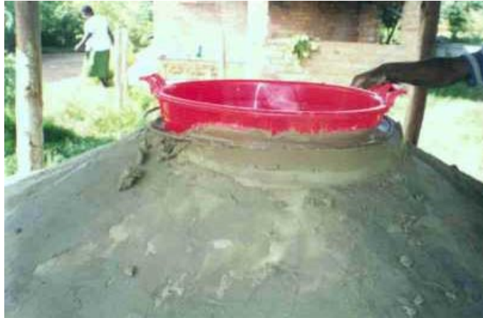
Figure 16 – showing the lip being built up around the basin – note the steel hoop in place
