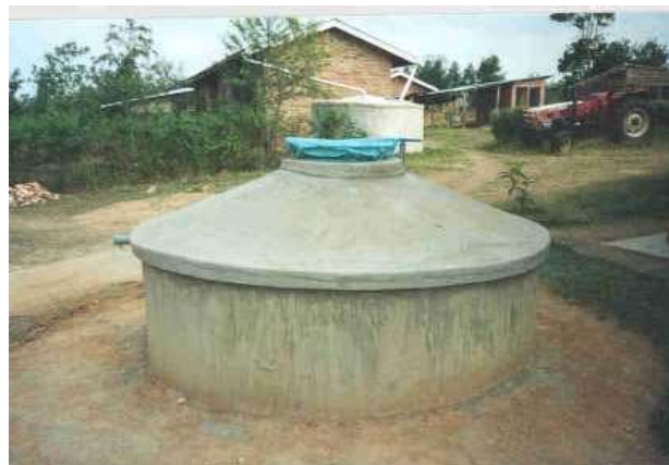
Figure 20 – A completed cover fitted on a partially below ground tank in Uganda
